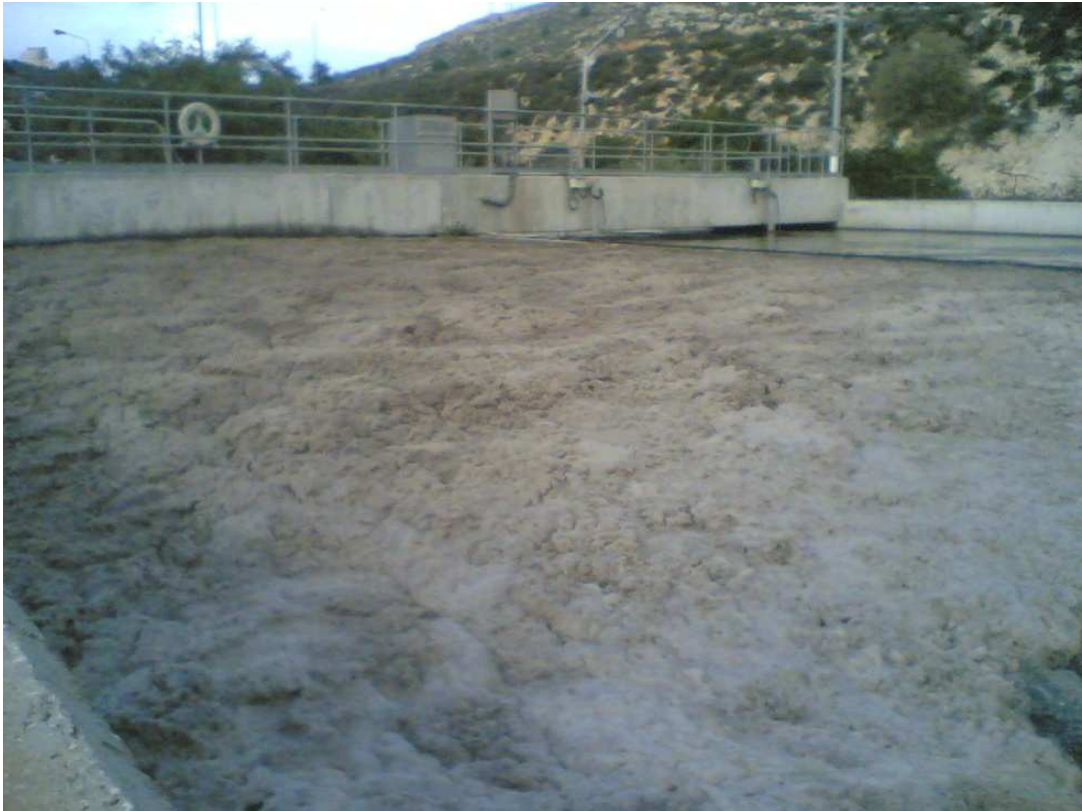
Figure 2. The foam in aeration tank (1) in AWWTP (April, 2010).
