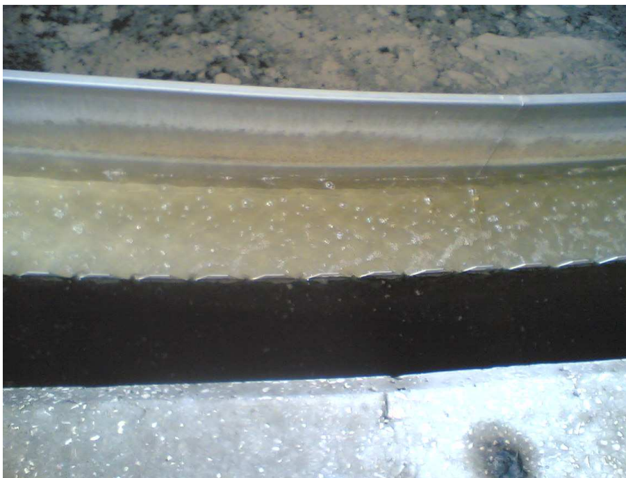
Figure 60. Turbid effluents from the sedimentation tank (2) (March, 2010)
