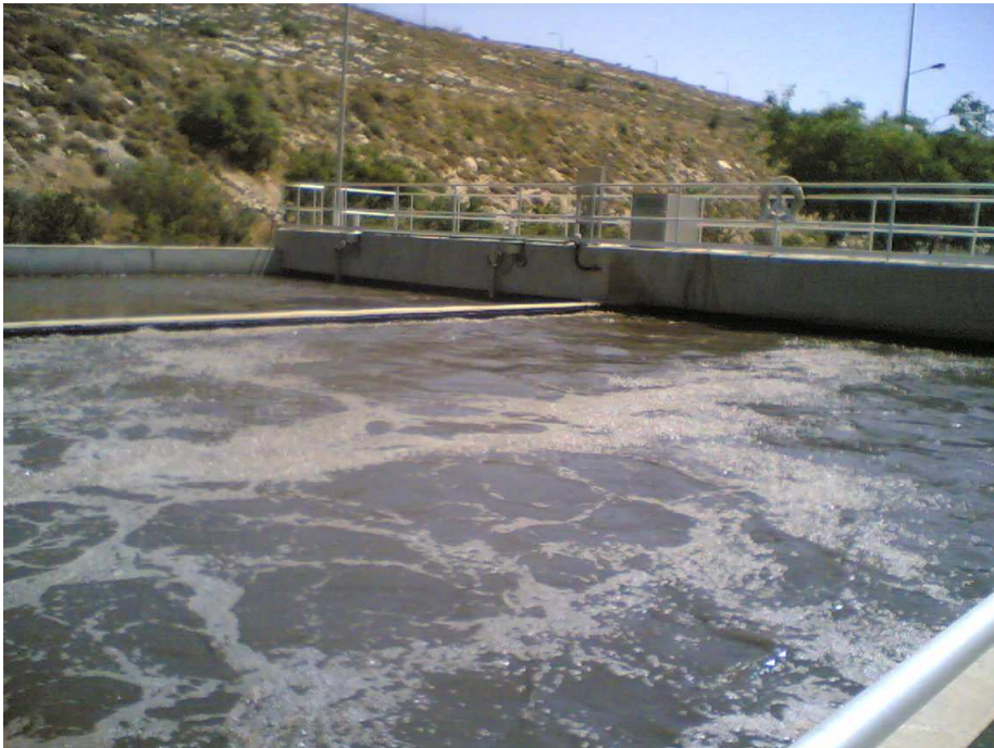
Figure 57. The aeration tank (1) in the summer (July, 2010)
