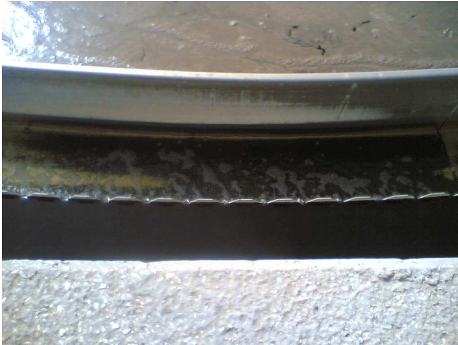
Figure 59. Turbid effluents from the sedimentation tank (1) (April, 2010)
