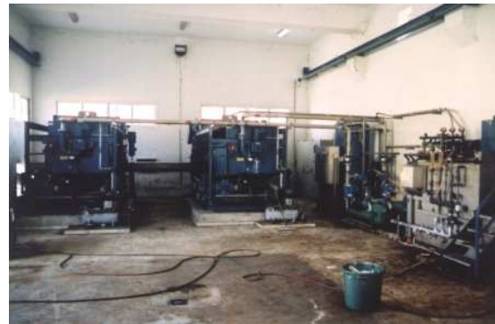
Figure 4b. Biosolids dewatering (Filter presses)
